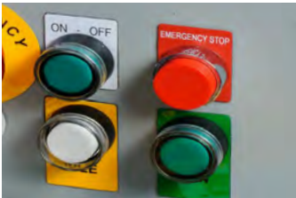
Control panel labels
