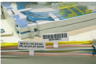
Fibre optic cable markers
